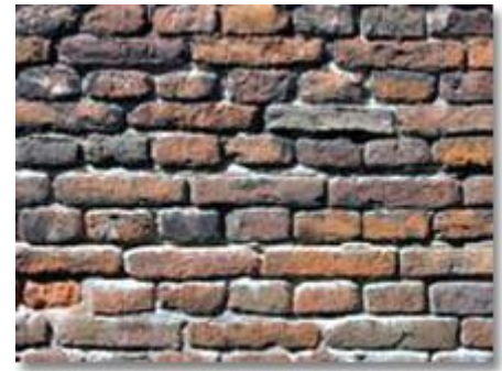
Sample; Worn brick wall.
